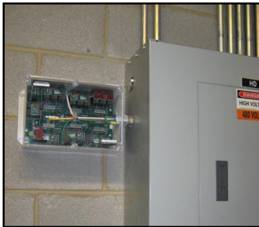
Surge Protection on Electrical Distribution Panel
