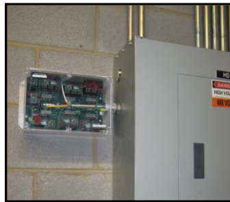
THOR SYSTEMS Series TSn Non-modular 150kA/Mode SPD fed by 3P 30A Panel Mounted Circuit Breaker (Clear Status Indication, NEMA 4X, Indoor or Outdoor Application)
