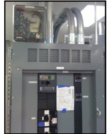
THOR SYSTEMS Series TSr 300 Modular SPD Mounted on Top of Service Entrance Switchgear
