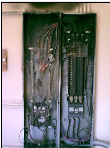
Results of SPD/TVSS Catastrophic Failure/Arc Flash
