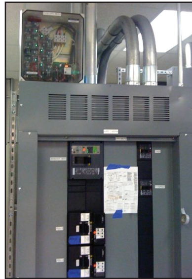
Modular Series TSr 300 (Mounted on top of Service Entrance Switchgear)
